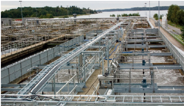
Himmerfjärden sewage treatment plant, Sweden
